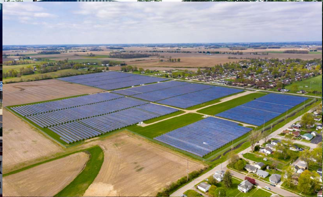
Manier Solar Field
