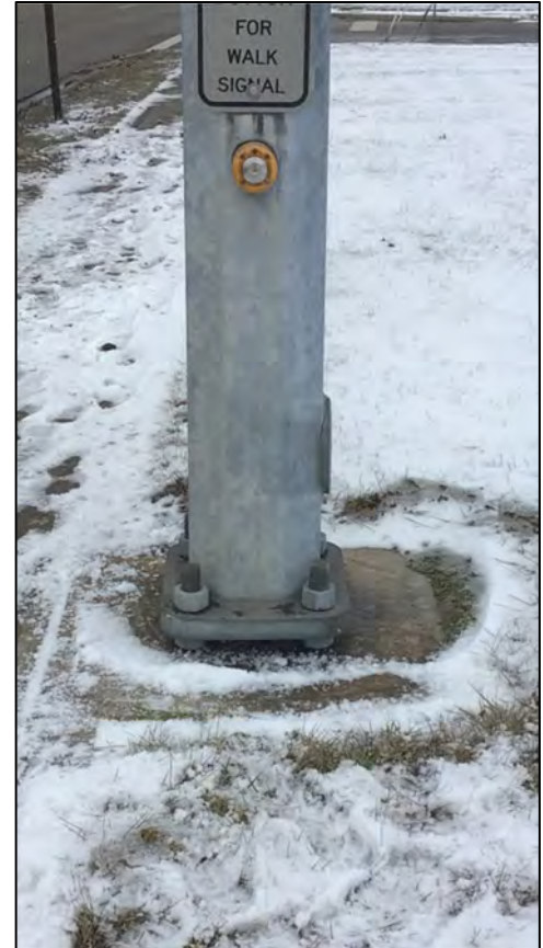
Example of pushbutton that has clear space within a lawn area and not on a compliant accessible route.
