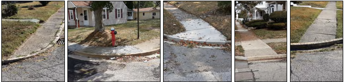
Examples of locations with PAR provided but no curb ramp is provided.
