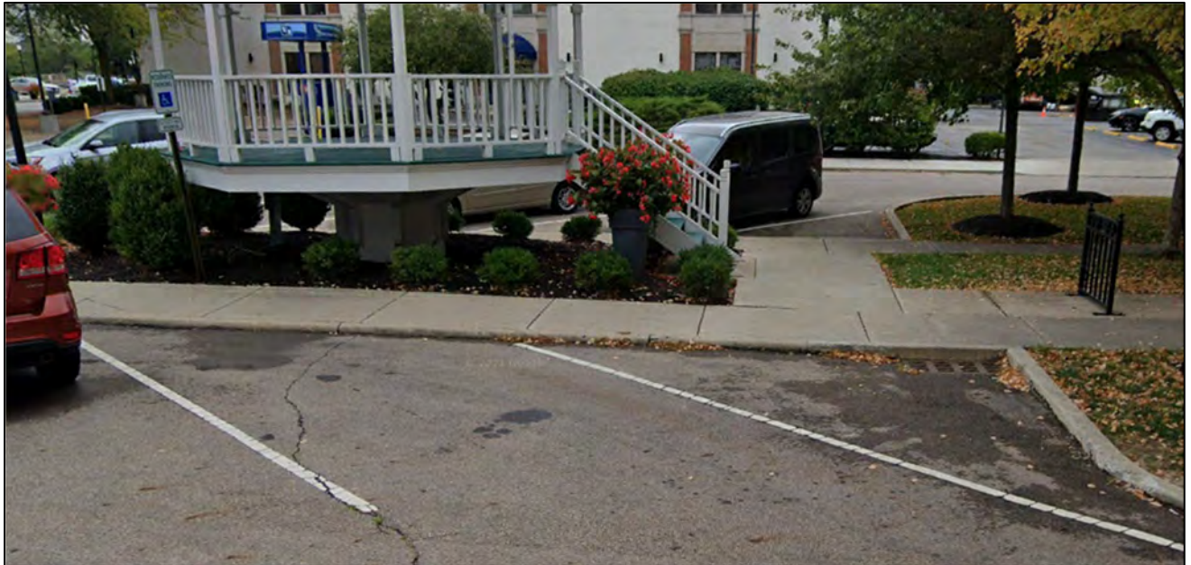
Angled on-street parking space with no compliant access aisle and no curb ramp available to access the PAR.
